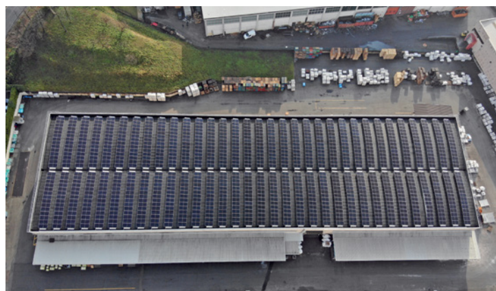
The rooftop photovoltaic system designed by Protesa
